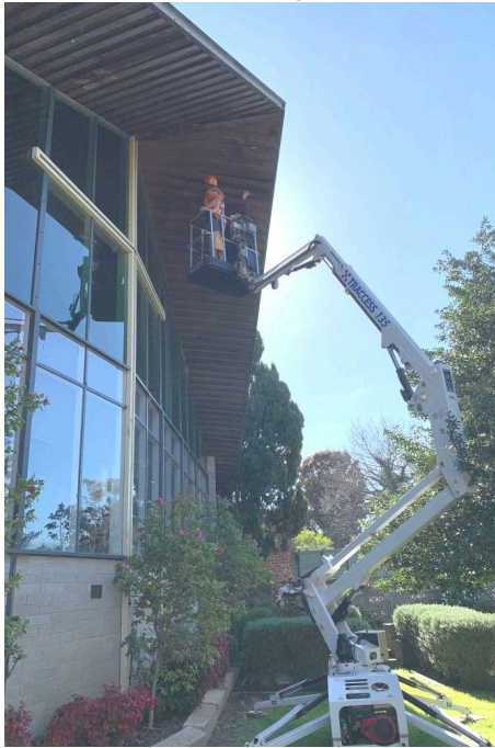
Glenn Farrington and his team have not only cleared the gutters at all our churches, but have also refastened the loose roof boards at St Andrew's.
